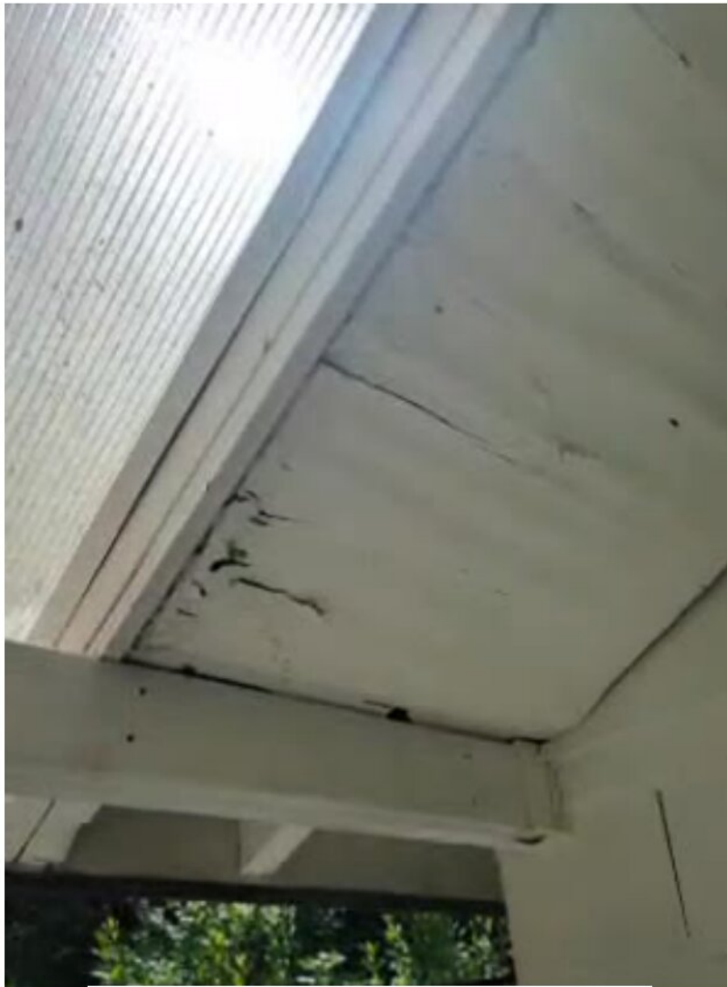
curled paint strips on soffit near beam junction
