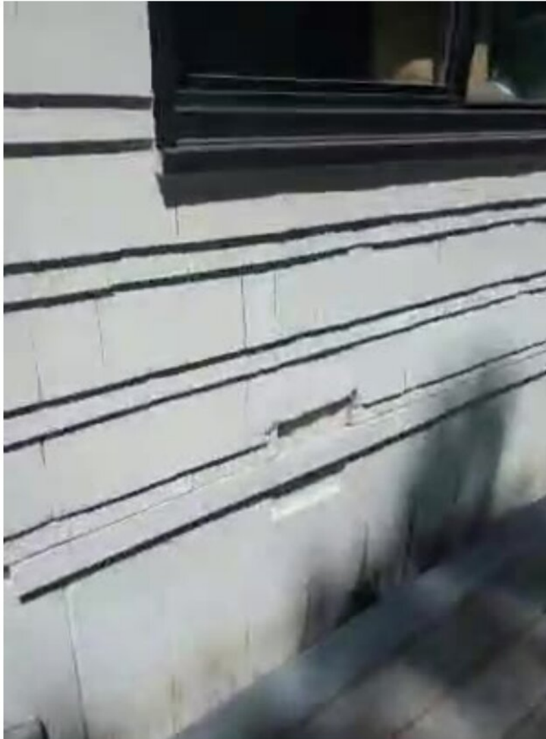
horizontal siding with cracking paint along joint lines
