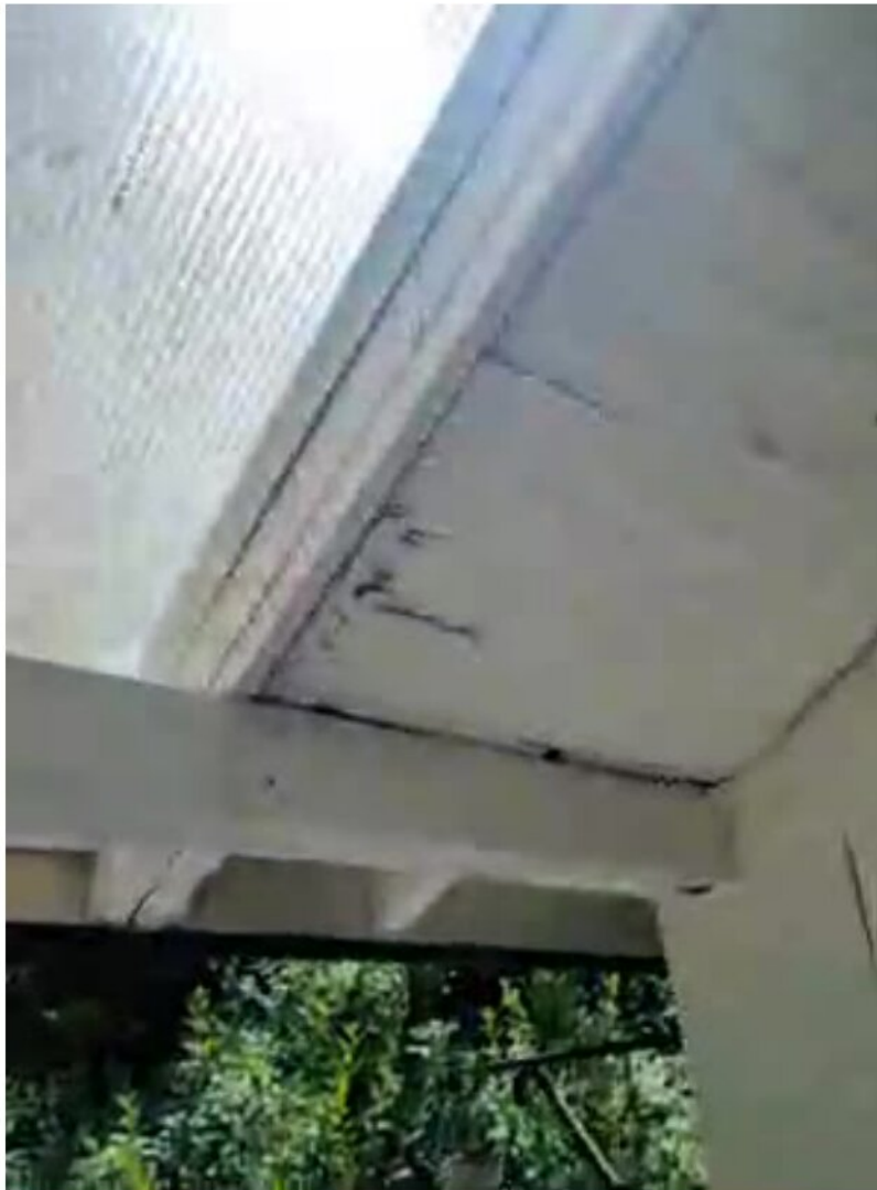
peeling paint along fascia underside
