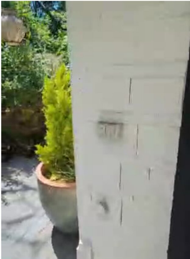
close view of column face with cracking paint
