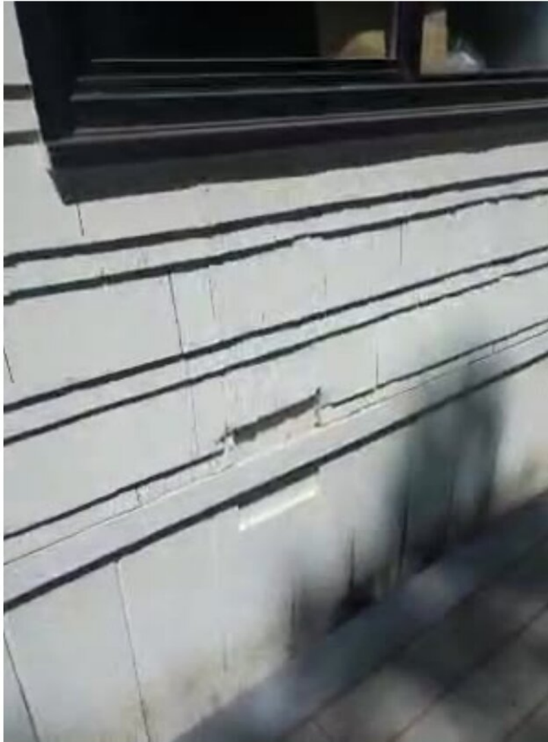
close view of cracked and separating paint on lower siding courses
