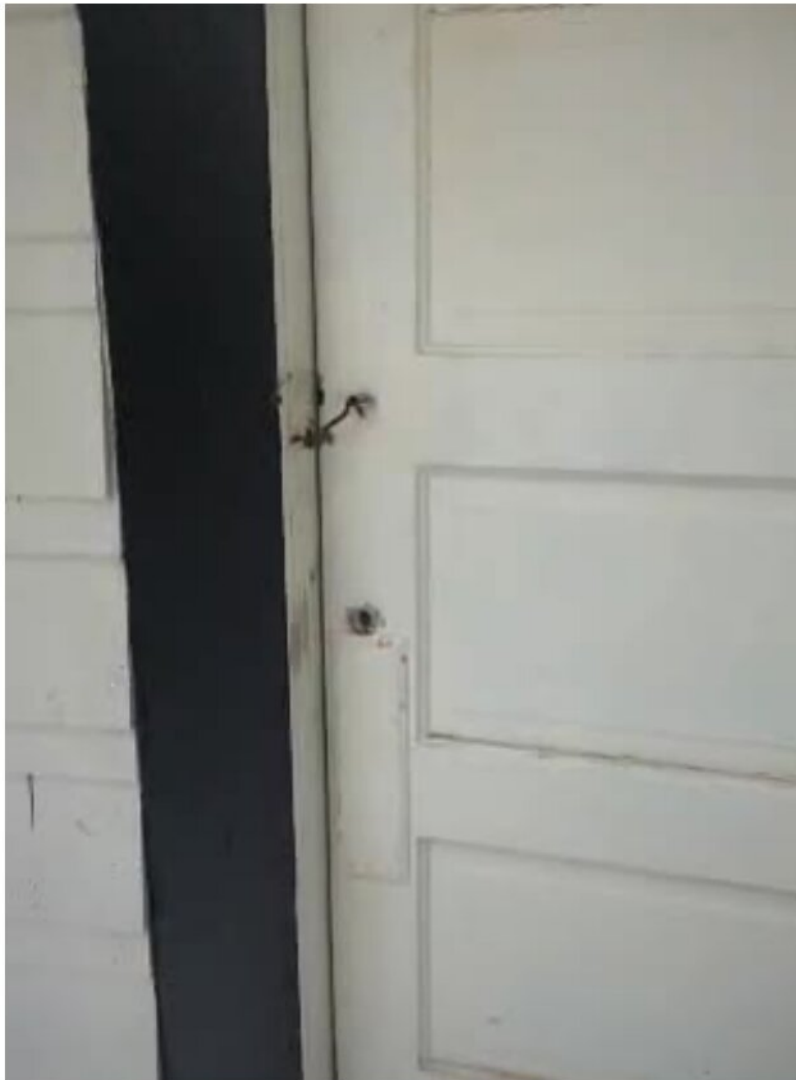
door edge showing latch and empty handle mounting hole
